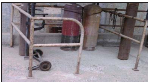
Figura 29: Central de Gases Topping 2
