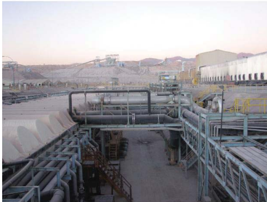
Figura 2-4. Vista general Tank Farm
